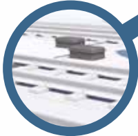
Cables for point machines
